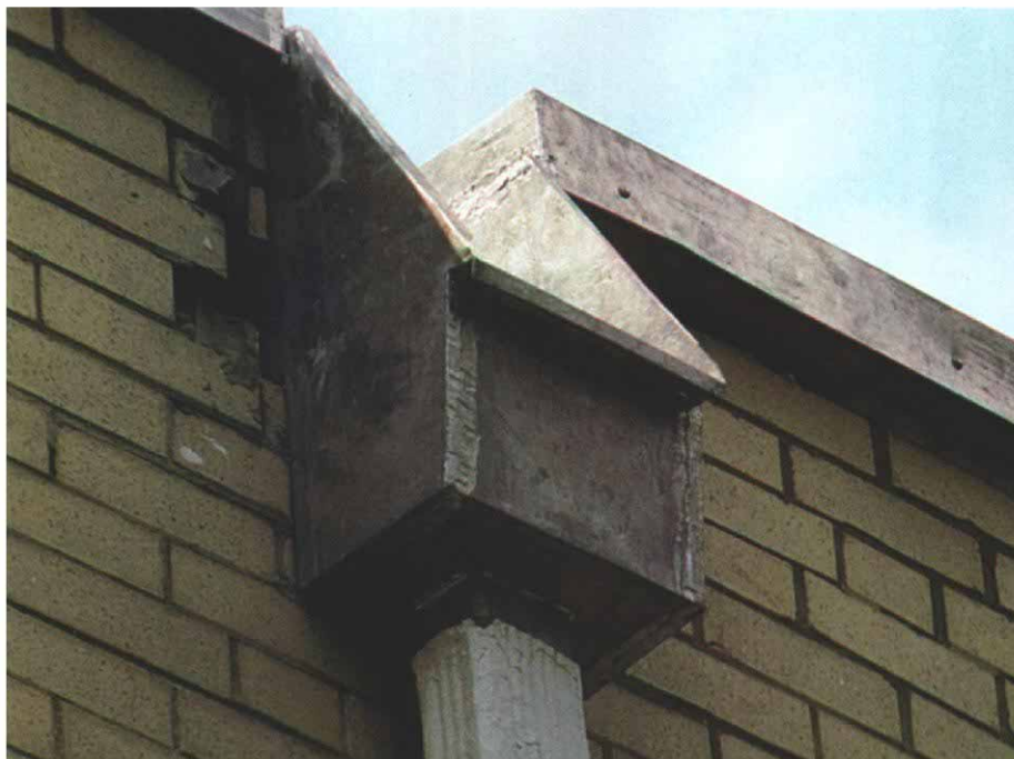
The parapet wall was opened wide to provide a substantial scupper. The photo above shows the completed parapet cap, scupper, and conductor head attached to the existing downspout.
