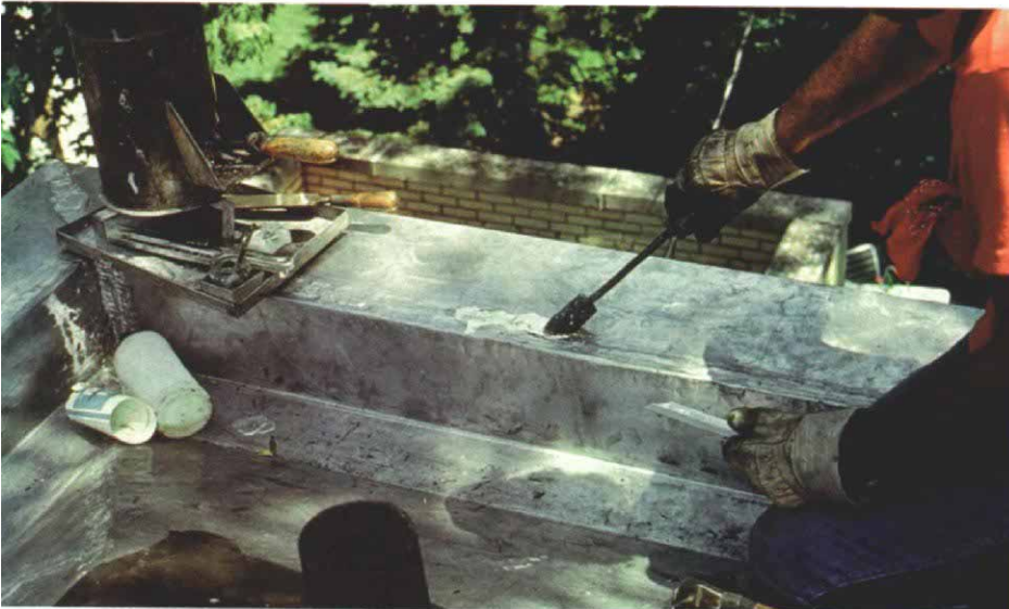
All seamed and overlapping joints of the gutter are soldered with 50/50 tin/lead solder. The charcoal-heated firebox shown above heats a soldering copper in its upper chamber. The lower container holds a jar of flux, a bar of sal ammoniac and bars of solder.
