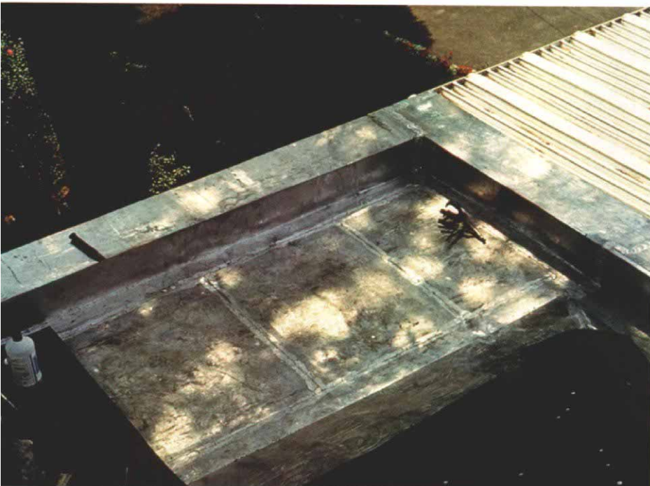
Two-ft. by 3-ft. lead-coated copper deck plates waterproof the flat-roofed wing of the house.
