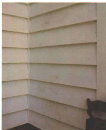
At inside corners, a square stick, usually \frac{3}{4} -in. by \frac{3}{4} -in., is nailed up and the clapboards butt into it.
