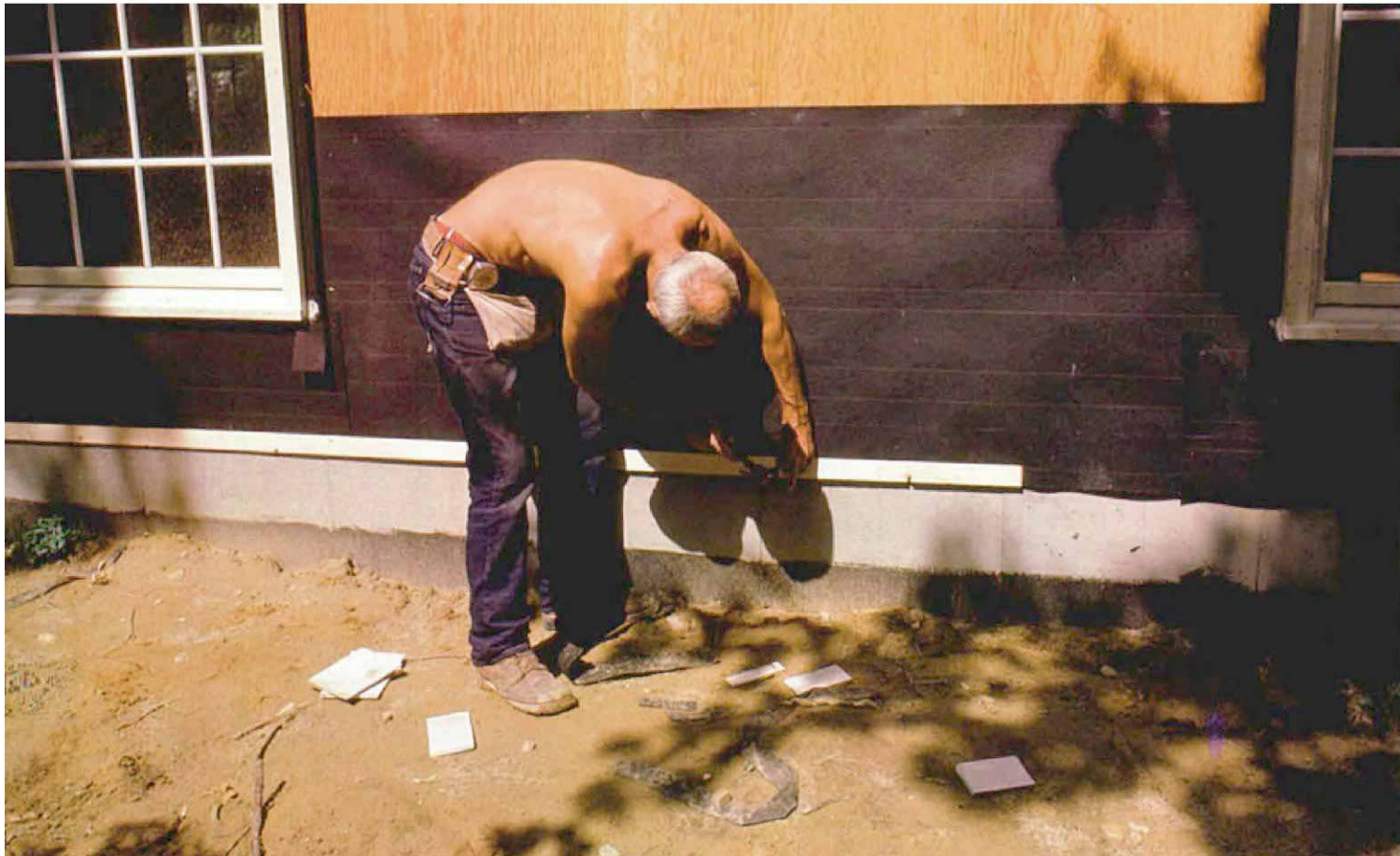
After the builder's felt is applied, a starter strip, representing the amount of overlap between courses, has to be nailed up so that the first course of clapboards will lay at the same angle as all the rest. Use 2-in. rippings from the top edge of the clapboards.
