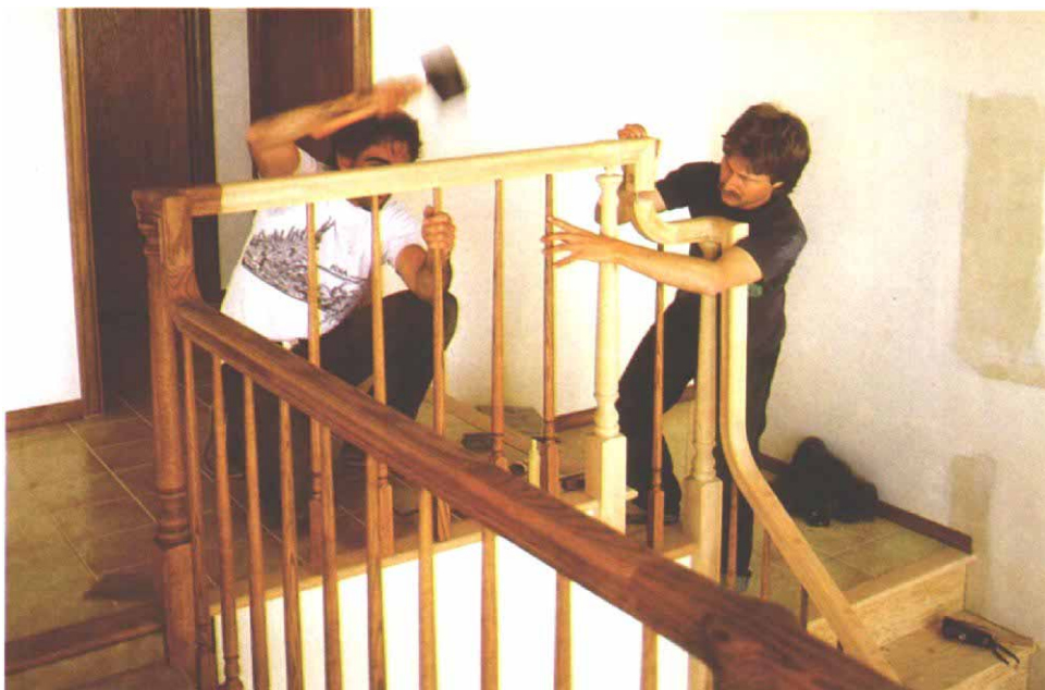
Lining up the balusters and worrying them into place for the final installation is a tricky job. It helps to have an extra pair of hands. Tapping with a rubber mallet ensures that the handrail and fittings are all the way down on the balusters and newels.
