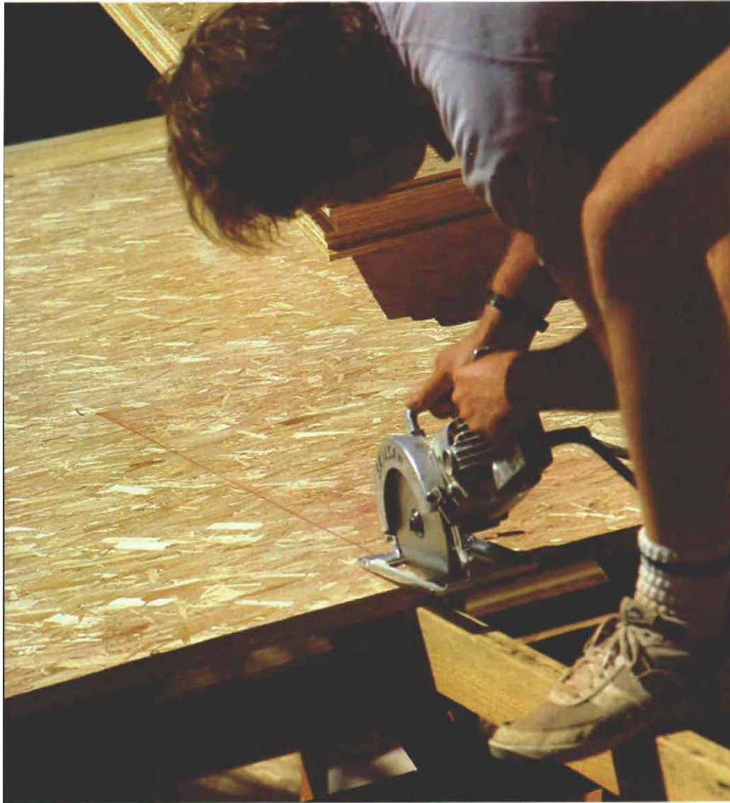
Cutting two pieces of roof sheathing at once eliminates tedious measuring and unwieldy rooftop cutting setups. Workers below should be warned about falling offcuts.
