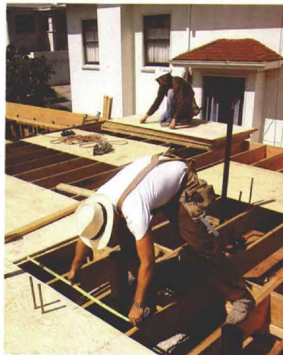
Try to work in pairs when laying out the bathroom subfloor. One calls out pipe centerlines while another marks their locations.
