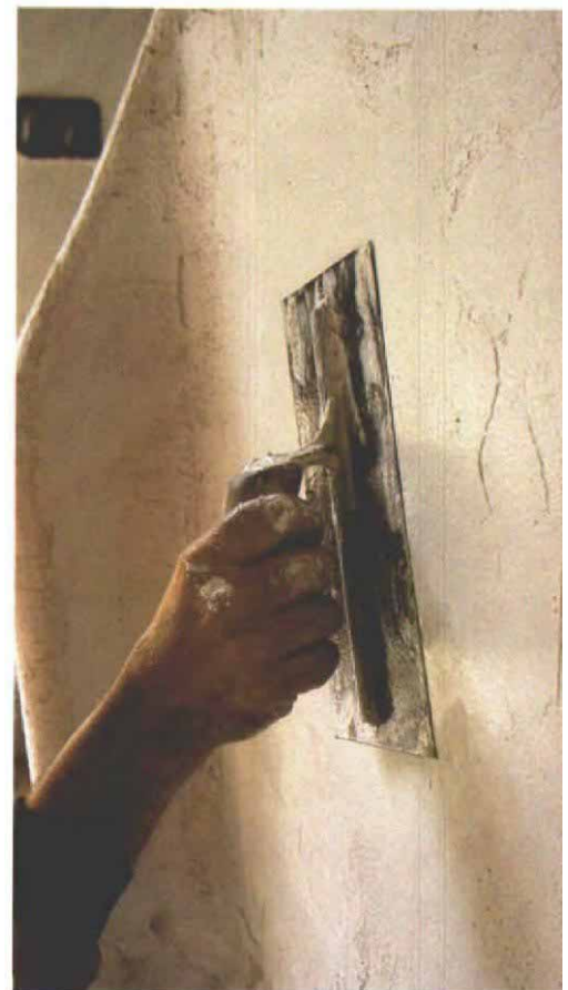
When the first coat begins to set up, it is worked with a notched trowel (left) to create shallow grooves, which provide a mechanical lock for the second coat of plaster.
