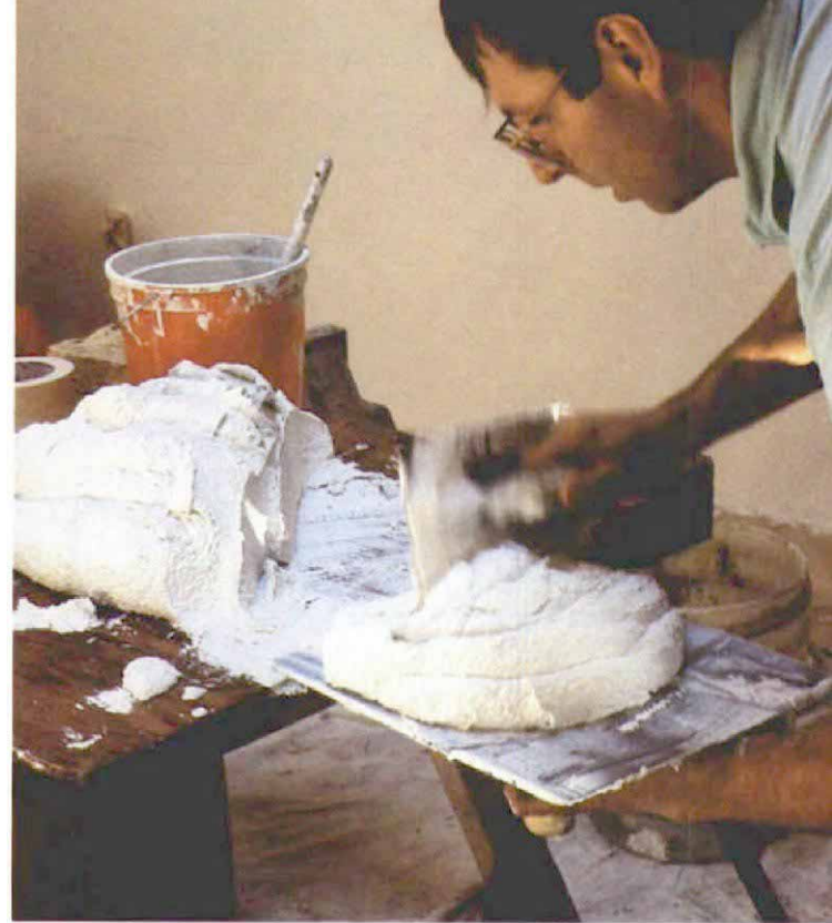
After mixing, the plaster is transferred to a work stand and a load is scooped onto a plasterer's hawk.
