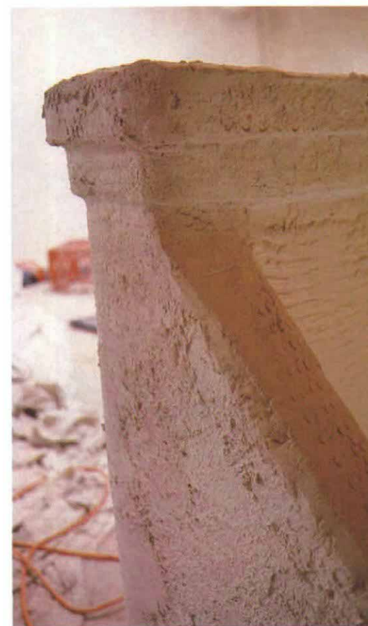
Metal lath can be used to reinforce outside corners and to anchor plaster to wood armatures. At top, the lath wraps around a low wall and over its 2x6 cap. From the other side (above), the wall begins to take on its finished shape after the first coat of plaster has been applied.
