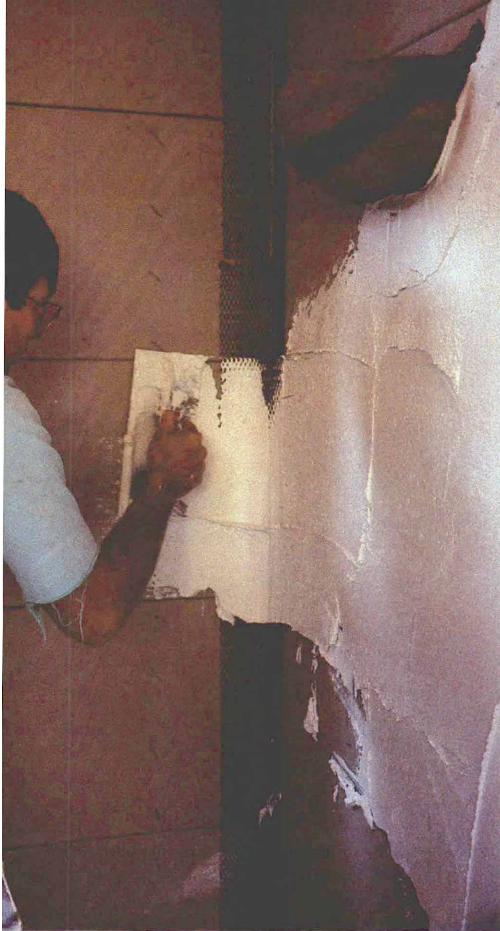
Radiused inside corners can be built up by nailing a narrow strip of rock lath into the corner, followed by a strip of metal lath. Here the author spreads the first coat of plaster across the wall to a depth of about \frac{1}{4} in. In the upper right-hand corner of the photo, a halved terra-cotta flower pot has been wired to the wall. It conceals a porcelain light fixture. The pot will eventually be plastered to appear as though it's part of the wall.
