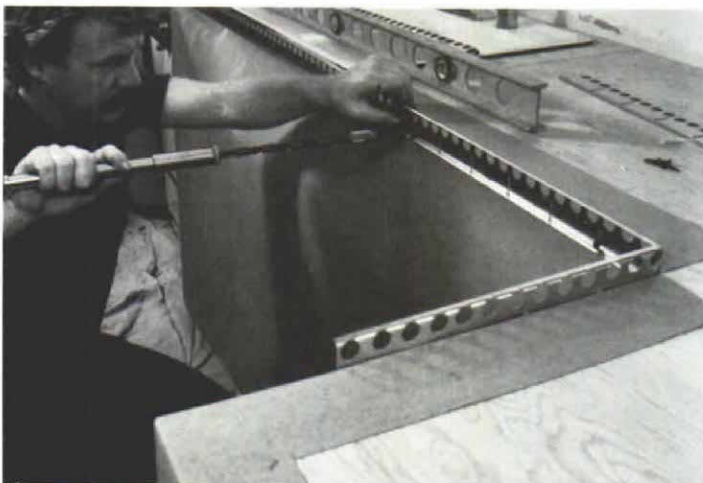
Sink rail. Before floating the mortar bed, Byrne screws a galvanized strip called a sink rail to the edge of the plywood substrate. It serves as a screed, edge reinforcement and a framework to anchor the thin layer of mortar that will face the edge of the countertop.
