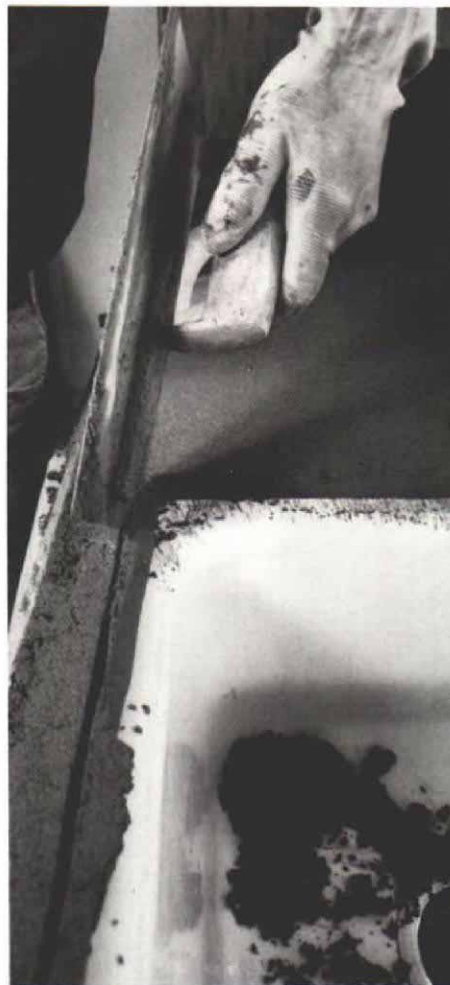
E. Edging. Before it hardens, any mortar that overlaps the sink rim is trimmed away. This allows the sink to be removed later if necessary, without damaging the mortar bed. The open edge will be trimmed with quarter-round tiles.
