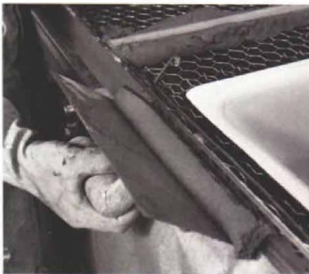
B. Wall mud —a special mortar blend that includes masonry lime and latex additive, which help the mortar to cling to vertical surfaces—fills the sink rail before the counter is floated. Some of this wall mud squeezes through the holes in the rail, keying it into the deck mortar.
