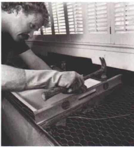
A. Float strips are the key to controlling the thickness of the mortar countertop. Here the author beds a float strip in a mortar pad, getting the strip's relationship to the sink rail right with a level. The float strips will guide the screed board while the mortar is leveled. Later, the strips will be removed and the resulting voids filled with mortar.
