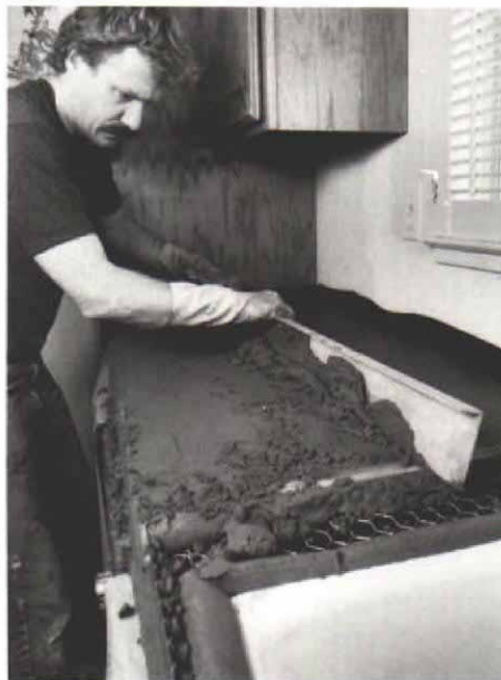
D. Leveling the deck mud. Byrne uses an aluminum straightedge as a screed board, and he moves it in a side-to-side motion as he gradually pulls it forward. Here both ends of the screed are resting on float strips. Note the difference in texture between the crumbly deck mud and the smoother wall mud used on the rail and around the sink.
