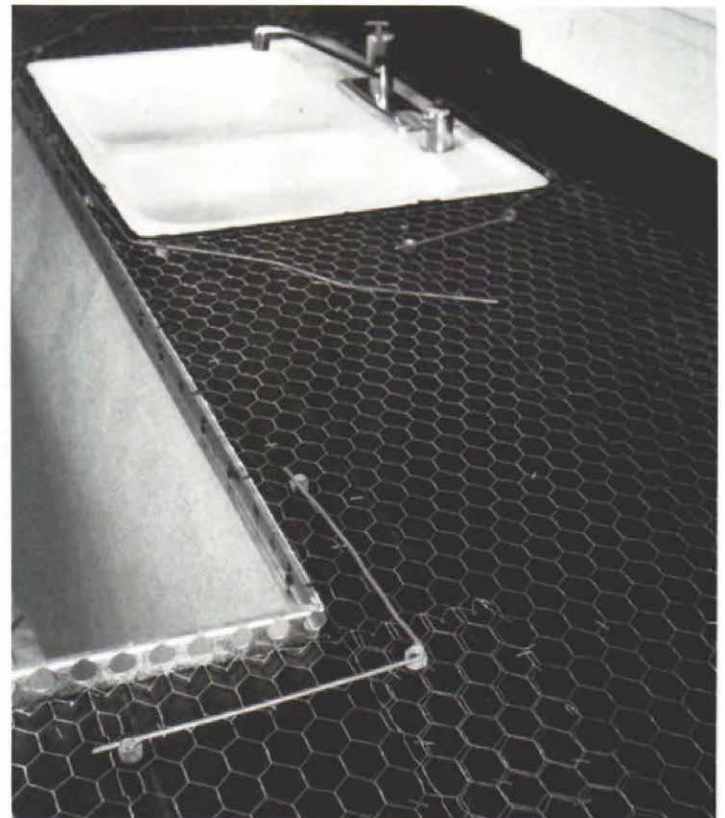
Reinforcement. Chicken wire stapled to the plywood substrate covers the area to be tiled. If a mortar counter cracks, it usually does so in the narrows around the sink, or at inside corners. These areas are reinforced with 9-ga. galvanized wire held in place by furring nails.
