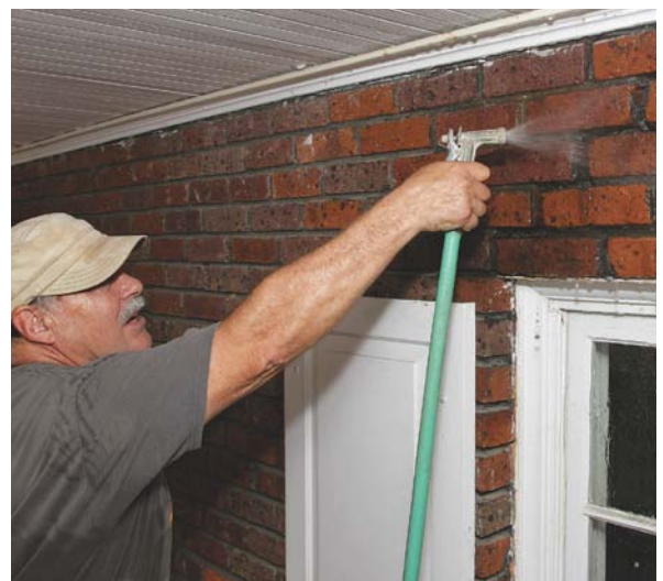
Dampen the area to be patched. Extremely dry masonry surfaces suck the moisture out of the mortar, preventing a proper cure. Spray the surface so that it's good and wet but not so that you inject a large amount of water behind the brick veneer. Let the surface dry so that the joints are still damp inside but there's no water on the surface of the bricks.
