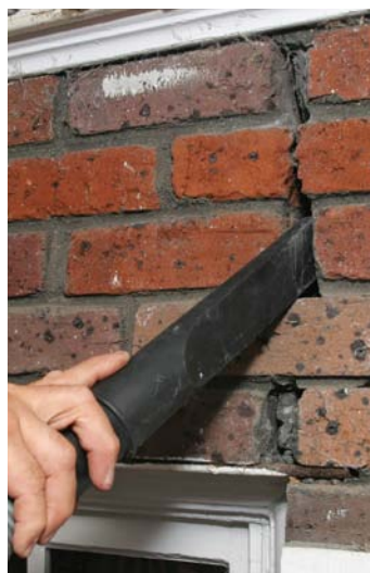
Vacuum out the loose material. The new mortar won't stick well to loose crumbs. Use a crevice vac attachment to reach deep into the joints.
