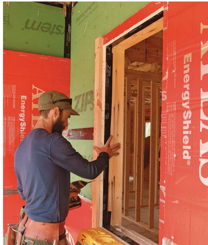
Install nailers. Screw rough-pine 5/4x3 nailers over the 1-in. foam to build the assembly out to the plane of the main 2-in. foam insulation.
