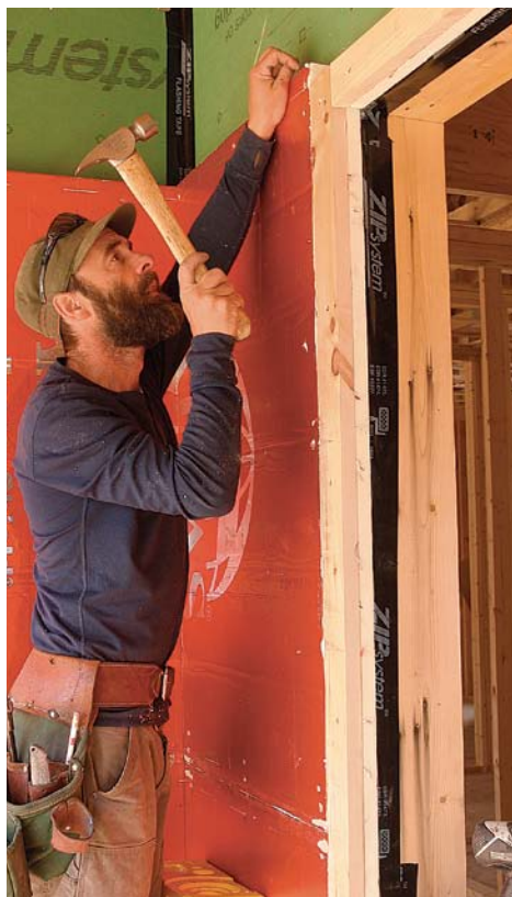
Butt the wall foam to the build-out. Installation of the rest of the insulation is simply a matter of cutting to fit and fastening with 2½-in. roofing nails.
