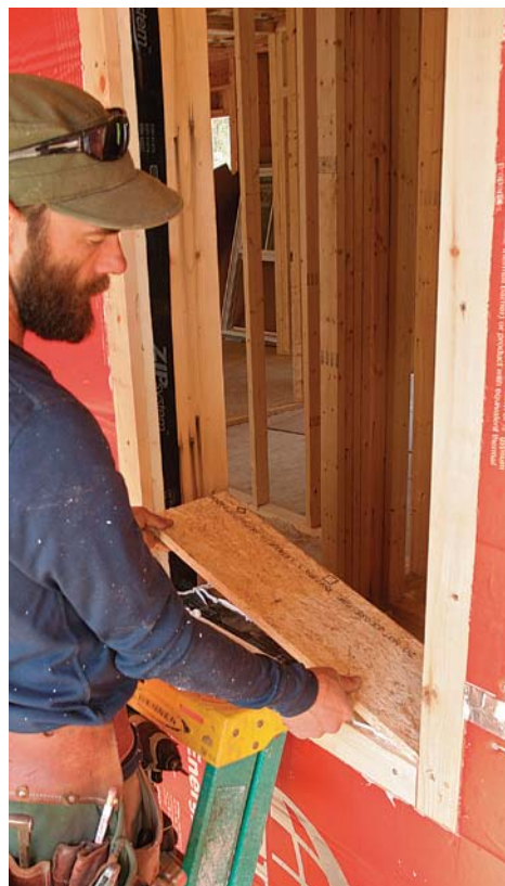
Add a solid sill. To create a base for windows and doors, fasten a piece of ¾-in. sheathing to the bottom of the rough openings.
