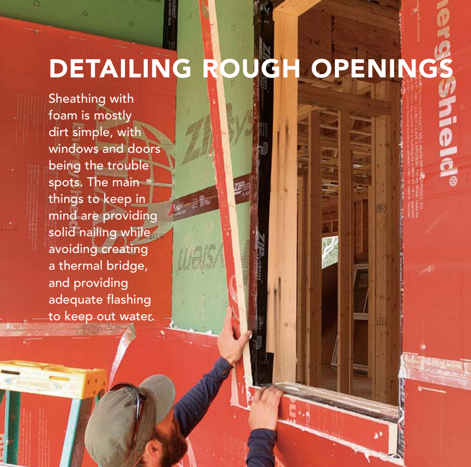
Create a thermal break. Nail foam strips 1 in. thick and 3½ in. wide around the opening.
