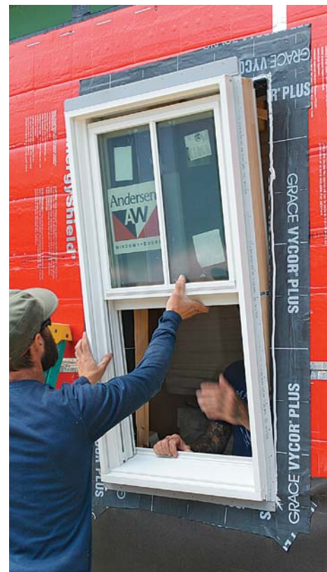
Proceed normally. With solid nailing established, installing windows or doors and integrating them with the WRB and the flashings is the same as on any other job.
