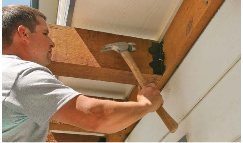
Nail the rafter to the ledger. Black-painted Simpson L70 angles connect the rafter and ledger. After installation, dings in the paint are touched up using an artist's brush.
