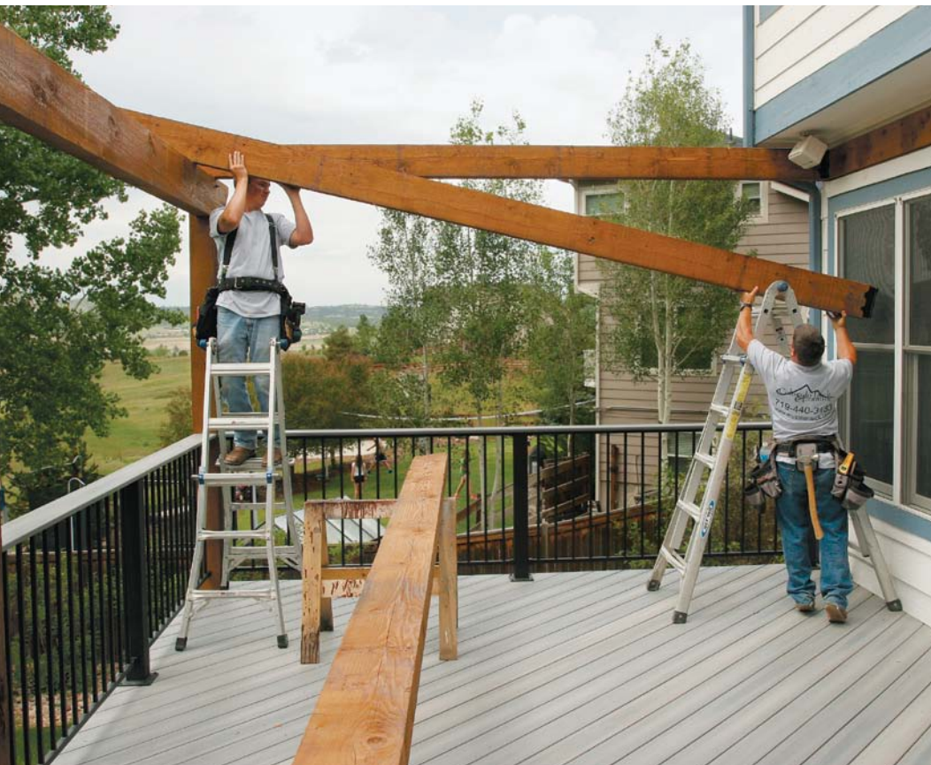
Raise the rafters in stages. The outer end of each rafter is placed on the beam, then the inner end is lifted into place.
