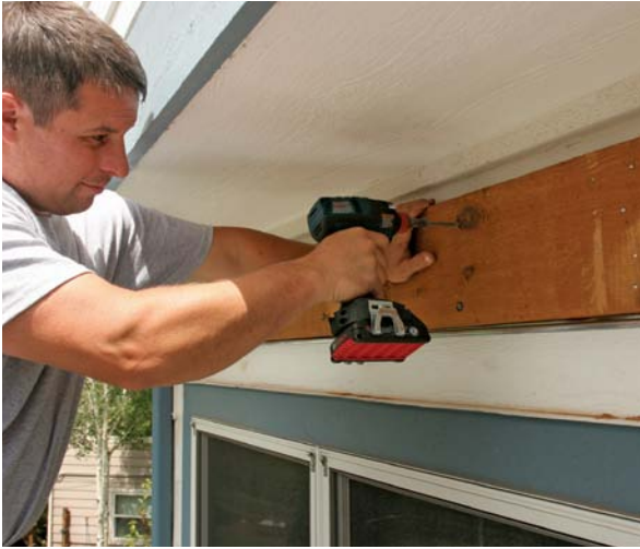
Screw the ledger to the house. A pair of 5-in. LedgerLok structural screws driven into each stud secures the rough-sawn 2x8 ledger to the house. LedgerLoks don't require pilot holes, as lags do.
