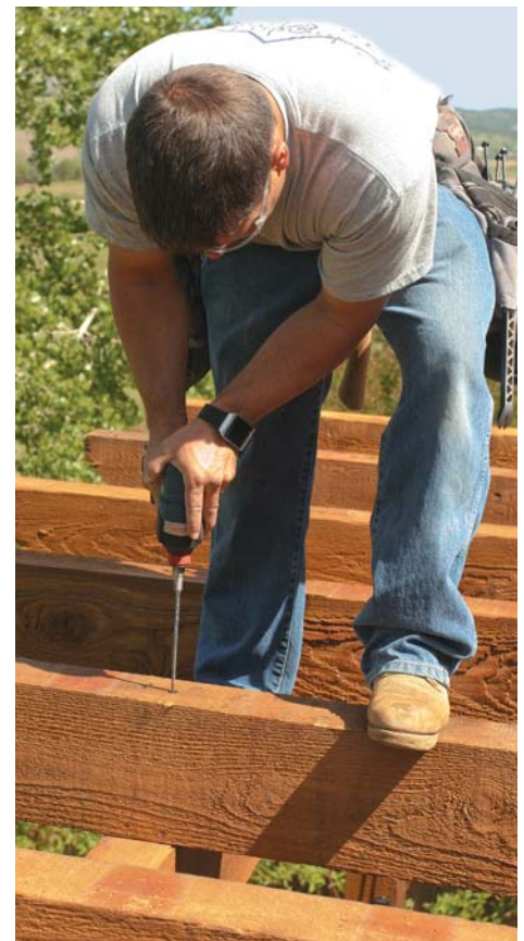
Screw the rafters down. Each rafter is held in place by two 10-in. TimberLok screws driven with an impact driver from above.
